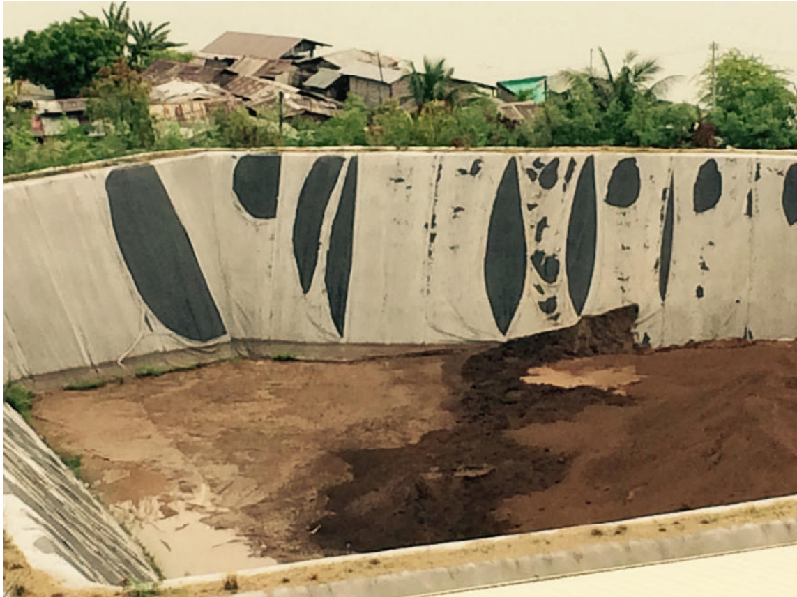
Figure: Emergency Ash Pond B at KSPC Compound with ash and showing damage to surface membrane
